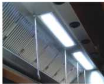
Exhaust Hood with Lighting arrangements
